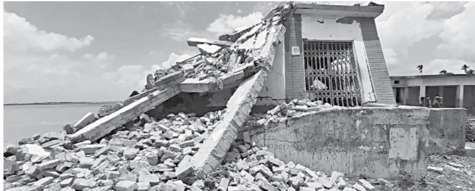
Paisha Majihail Government Primary School at Solimabad in Tangail's Nagarpur lies ravaged due to erosion by the Jamuna river on Sunday. Above, a scene of erosion by the Brahmaputra at Dhanarchar Nutangram village of Jadurchar union in Kurigram's Roumari upazila. PHOTO: STAR
