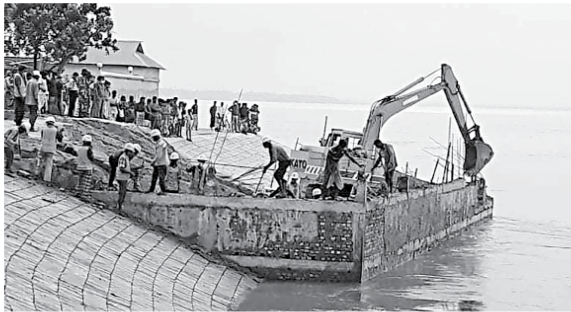
Workers engaged by Kalihati upazila administration dismantling a permanent structure constructed illegally on a village protection embankment along the Jamuna in Gorilabari village of the upazila.
