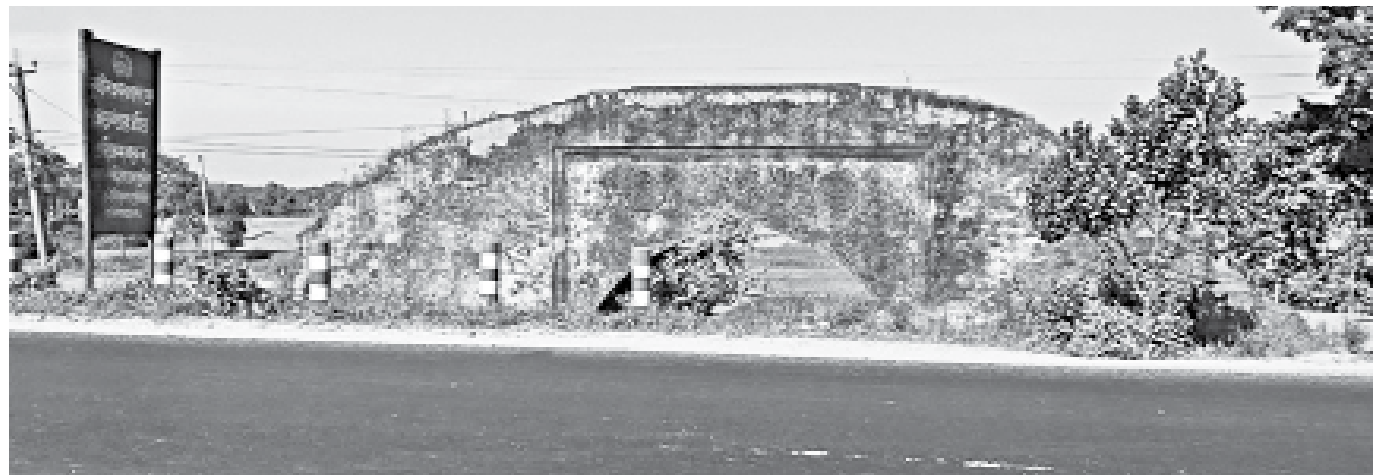
Roadside view of the century old bridge, locally called Hatirpool, on the north side of Dhaka-Sylhet highway at Bariura village in Brahmanbaria's Sarail upazila. PHOTO: STAR
