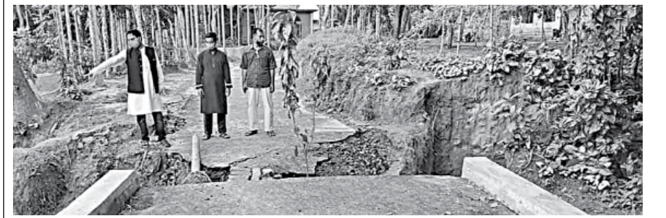
A one kilometer road from Gourangi Uttar Para to Akashi School in Tangail's Ghatail upazila gets damaged within days of its construction.
