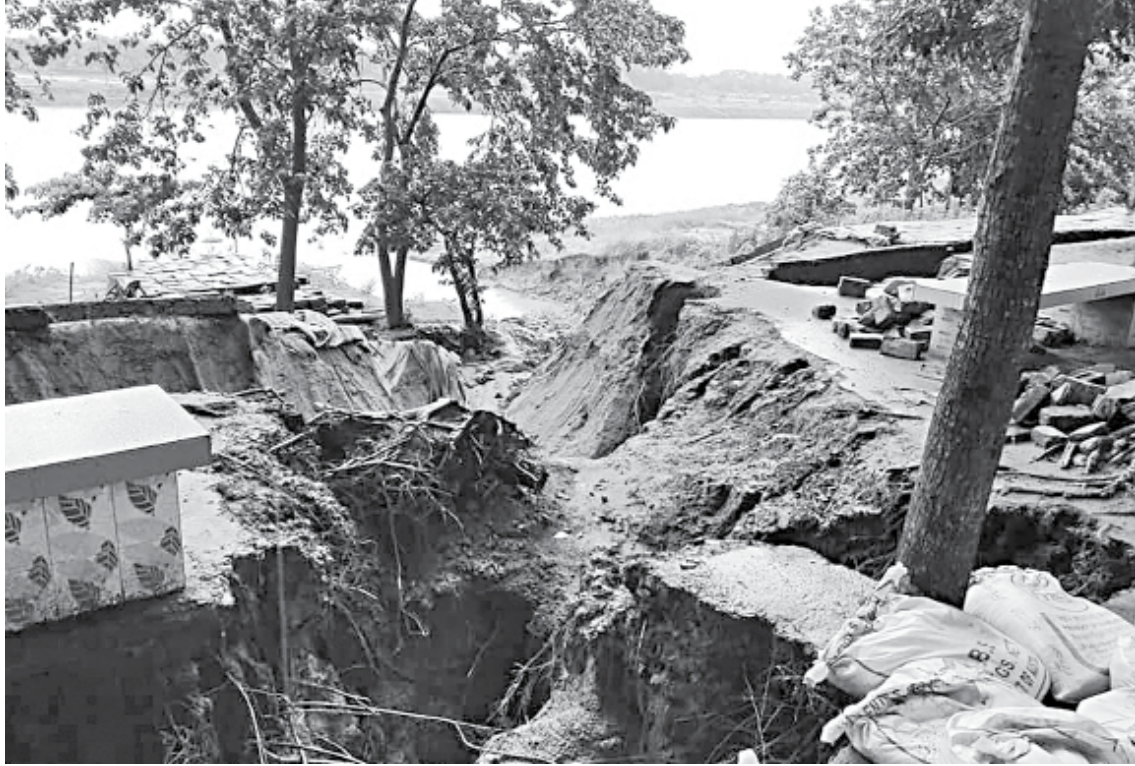
This area of Mymensingh City Protection Embankment, along with a few other spots, developed breaches following last week's heavy downpour.
