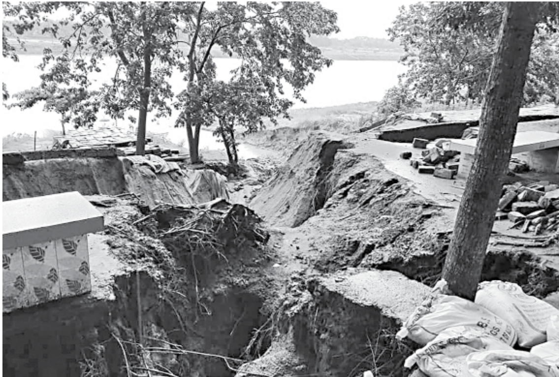
This area of Mymensingh City Protection Embankment, along with a few other spots, developed breaches following last week's heavy downpour.
