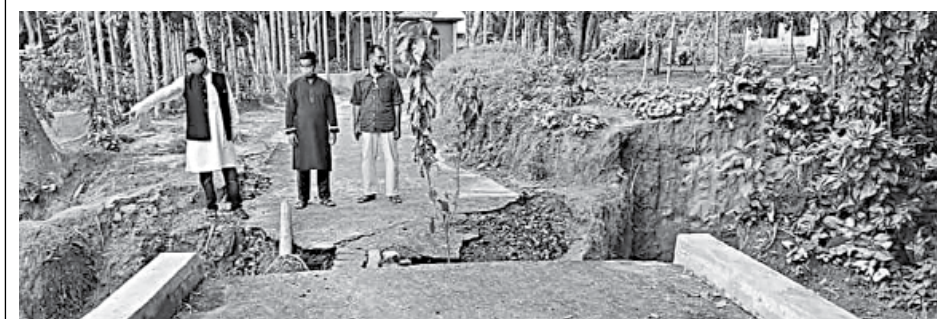
A one kilometer road from Gourangi Uttar Para to Akashi School in Tangail's Ghatail upazila gets damaged within days of its construction.
