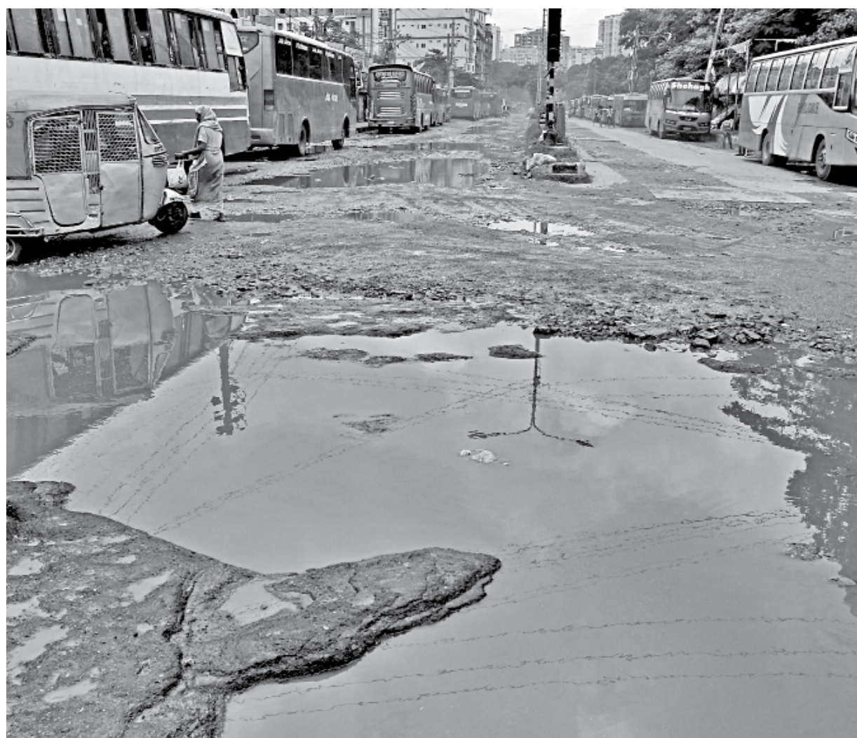
This road at the capital's Motijheel has remained dilapidated for the last few months. With frequent rain recently, water has been collecting in the potholes, causing pedestrians and vehicles to deal with an even worse situation. This photo was taken yesterday.
