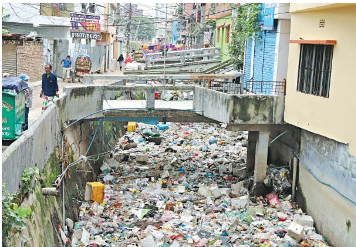
Encroachment and throwaway plastic goods make it seem like Segun Bagicha canal in the capital's Manda is a stream of garbage. The clogged canal may cause flooding in the area during monsoon. The photo was taken yesterday.
