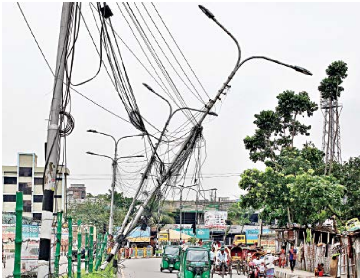
AN ACCIDENT WAITING TO HAPPEN... A few streetlights near Kamalapur Inland Container Depot (ICD) are precariously leaning over electric wires, as last weekend's heavy storm left a few casualties around town. The photo was taken on Friday afternoon.
