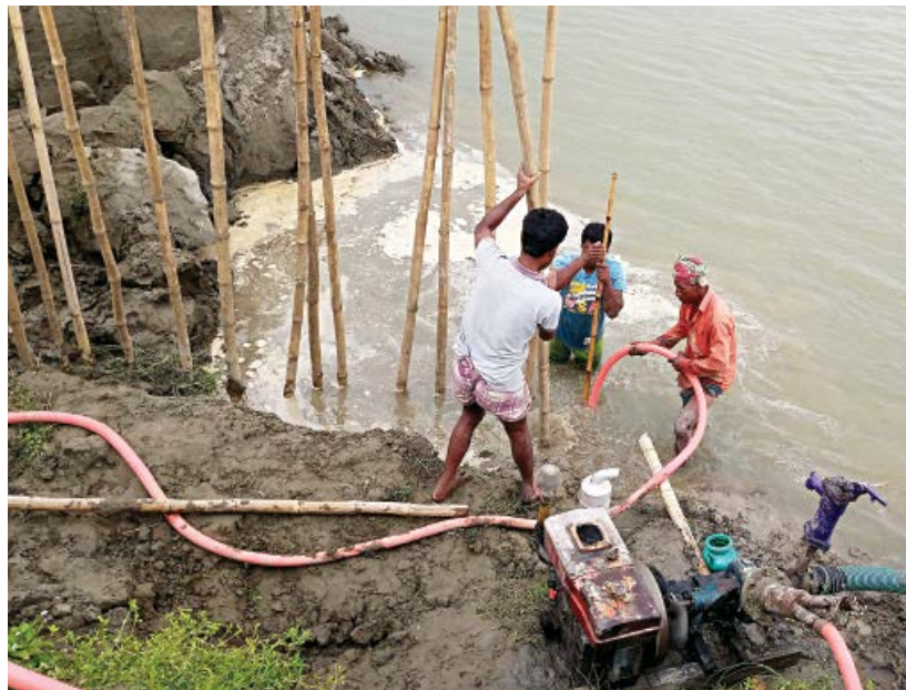
Locals engaged in bamboo piling work at Char Sajai village of Kodalkati union in Kurigram's Rajibpur upazila.
