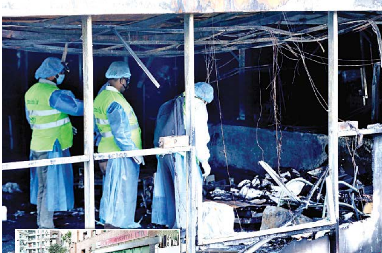
CID officials inspect charred remains at the isolation coronavirus unit of the capital's United Hospital yesterday. Inset, the temporary unit, which was set up outside the hospital's main building. Five patients being treated at the unit were killed after a devastating fire broke out there on Wednesday night.
