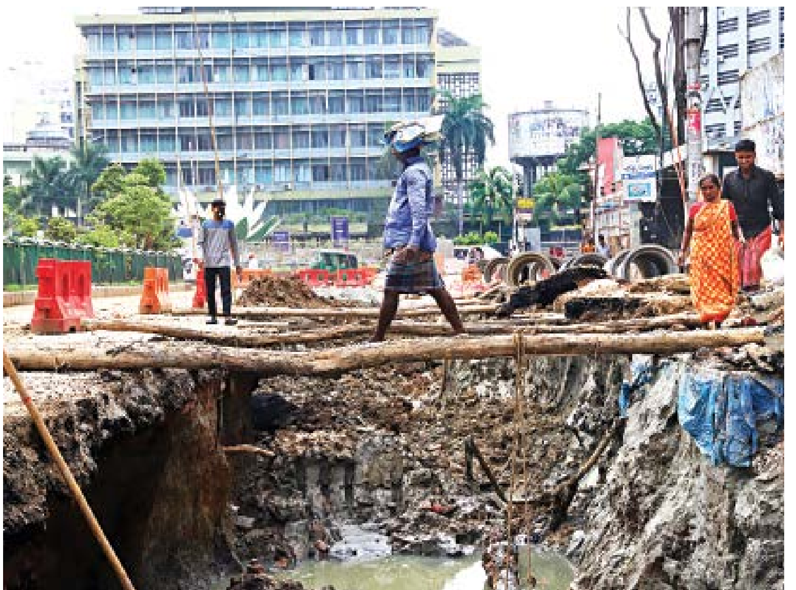
Large portions of a road leading to Shapla Chattar in the capital's Motijheel have been dug up, as sewage work continues there for the metro rail project. At any other time, this would cause a serious headache for commuters on one of Dhaka's busiest roads, but thanks to the general holiday, that has not been the case. The photo was taken earlier this week.
