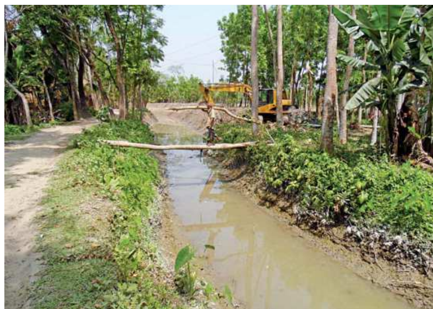
Re-excavation work of Mathbari canal in Jhalakathi's Rajapur upazila has begun recently.
