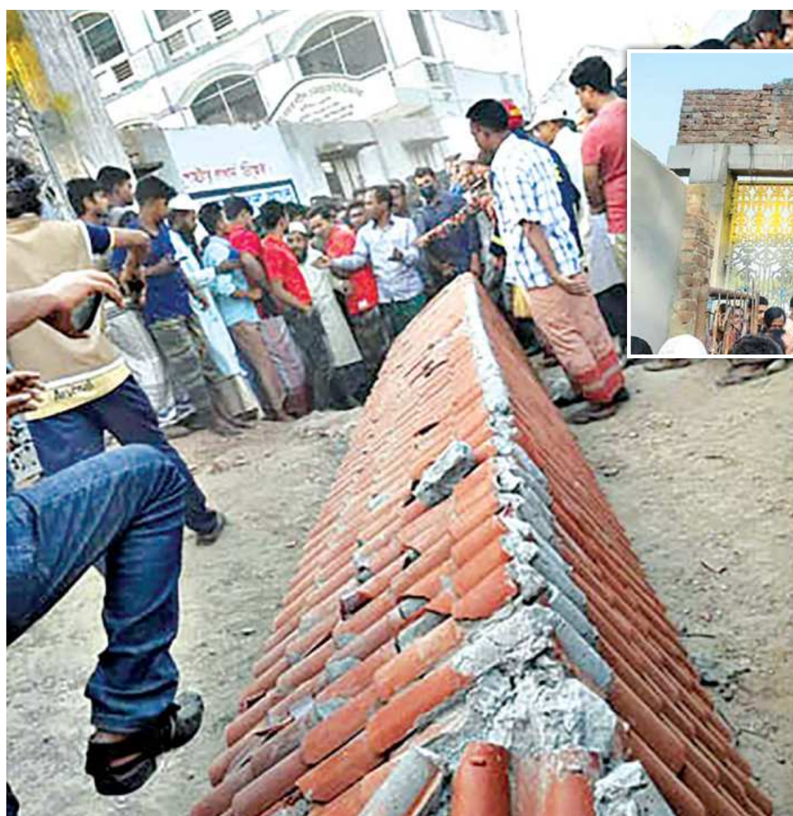
This large chunk of an under-construction college gate, inset, in Tarash upazila of Sirajganj fell yesterday killing four people and injuring 10 others. Shoppers at the nearby Gulta Bazar were standing beneath the gate for shelter when it collapsed and killed three on the spot, while another victim died on way to the hospital.
