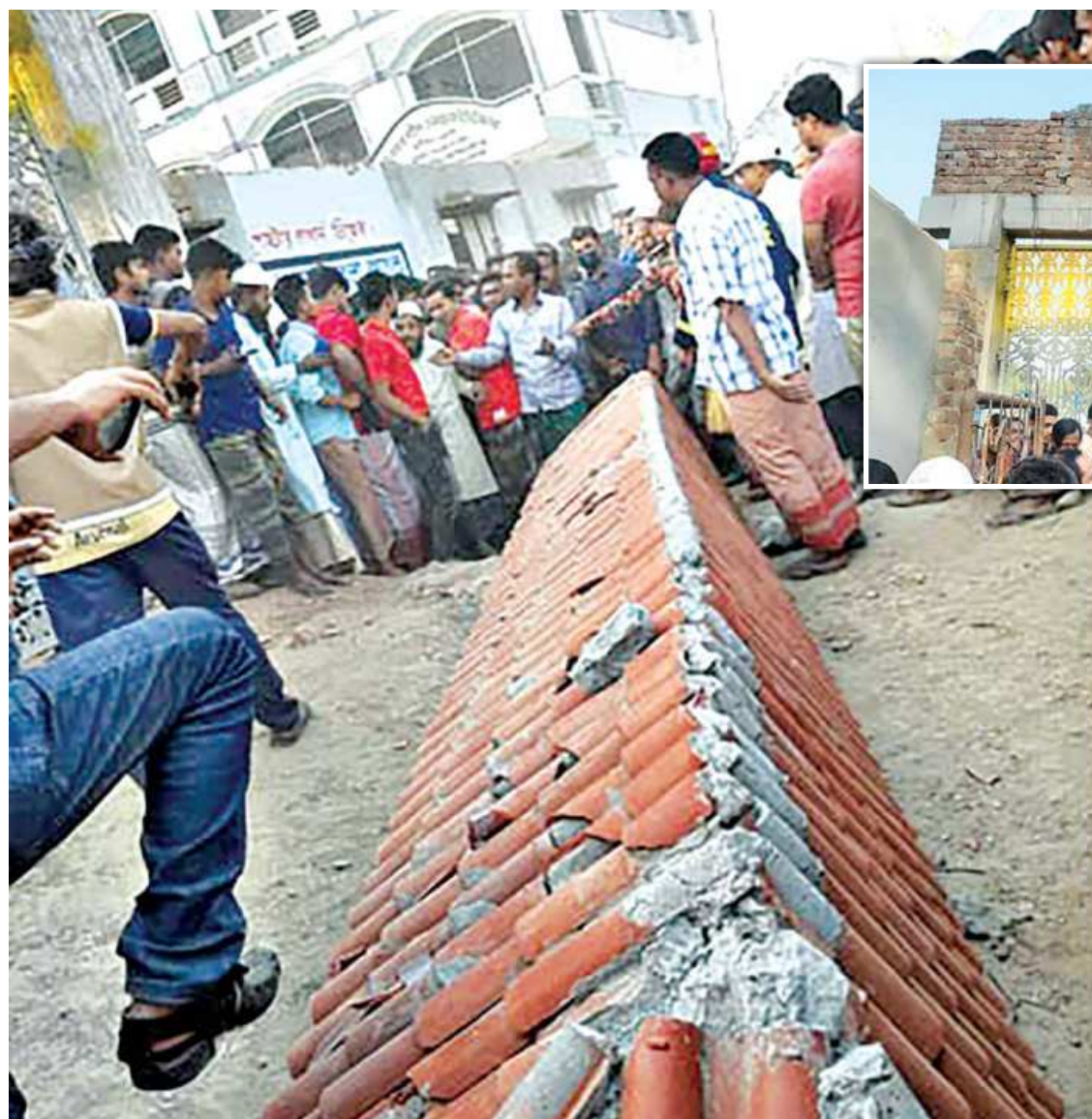
This large chunk of an under-construction college gate, inset, in Tarash upazila of Sirajganj fell yesterday killing four people and injuring 10 others. Shoppers at the nearby Gulta Bazar were standing beneath the gate for shelter when it collapsed and killed three on the spot, while another victim died on way to the hospital.
