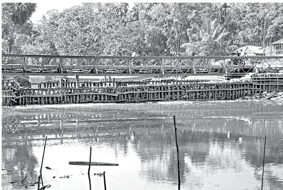
A group of local people build an illegal dam in Varani Khal of Barishal's Bakerganj upazila to stop erosion by river.
