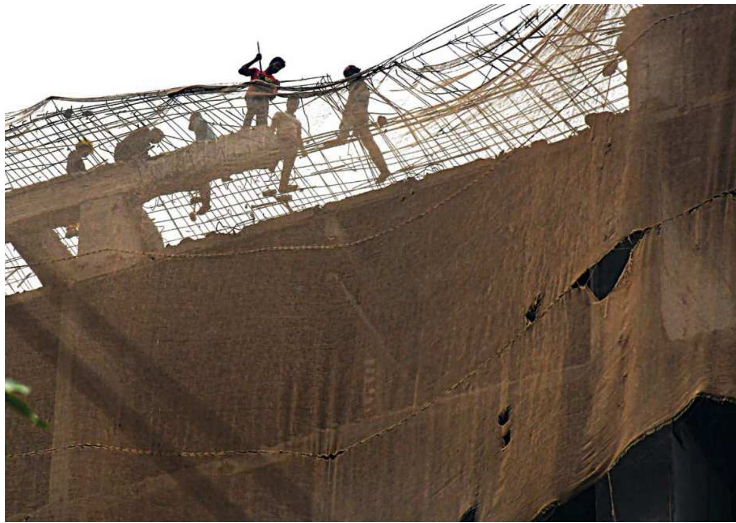
With no safety gears on, workers knocking down the BGMEA Bhaban, illegally built on Hatirjheel, in the capital's Karwan Bazar area yesterday. Their disregard for safety puts them at risk.
