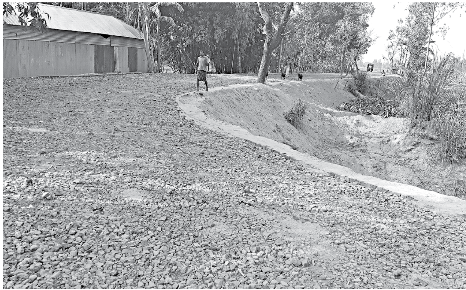
Poor quality brick chips instead of first class brick chips have been used for widening a 6.24km long road stretching from Sadar upazila's Mogholhat area to Aditmari upazila's Durgapur area in Lalmonirhat.
