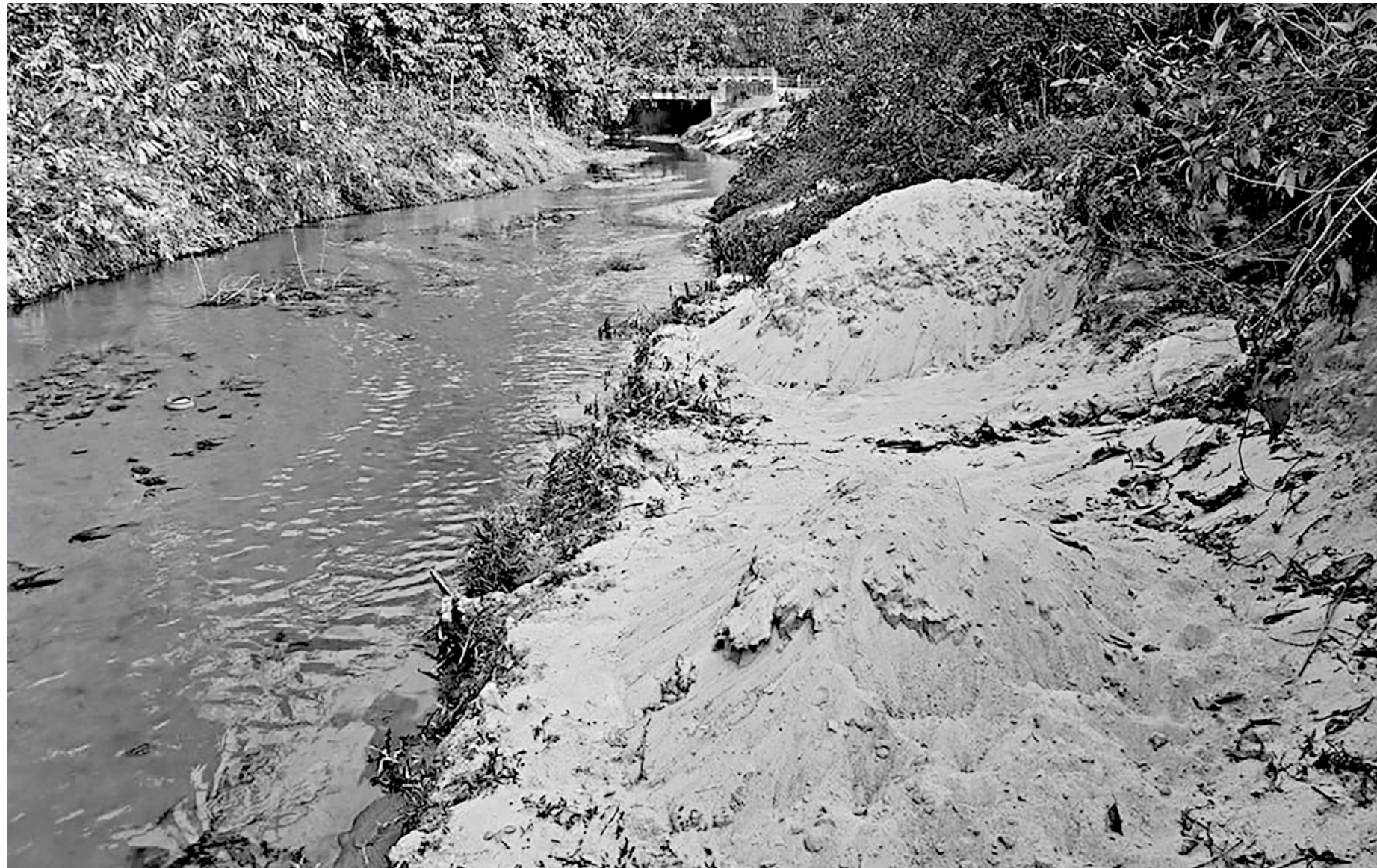
Extraction of silica sand from within 500 metres of this railway bridge over the Barachhara canal in Kulaura upazila of Moulvibazar poses threat to the important structure on Sylhet-Dhaka route. A nearby road bridge (not in the picture) also faces risk due to the unscrupulous act.
