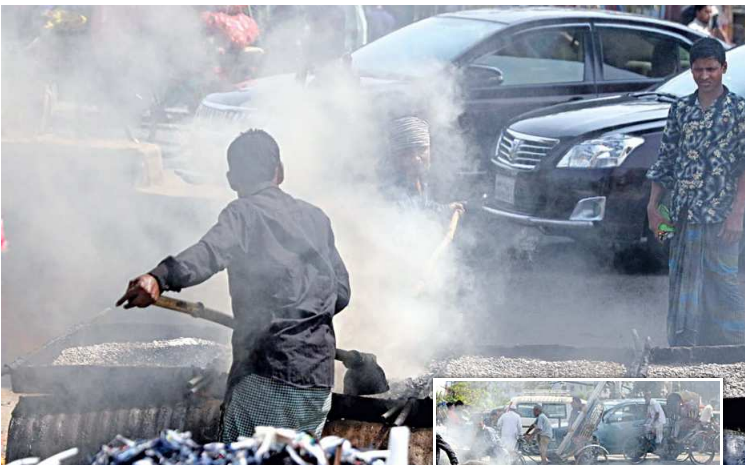
Discarded plastic, inset, being used as fuel for a makeshift burner to heat tar and stone chips for road repair. The toxic fume engulfed the area near the FDC level crossing in the capital yesterday.
