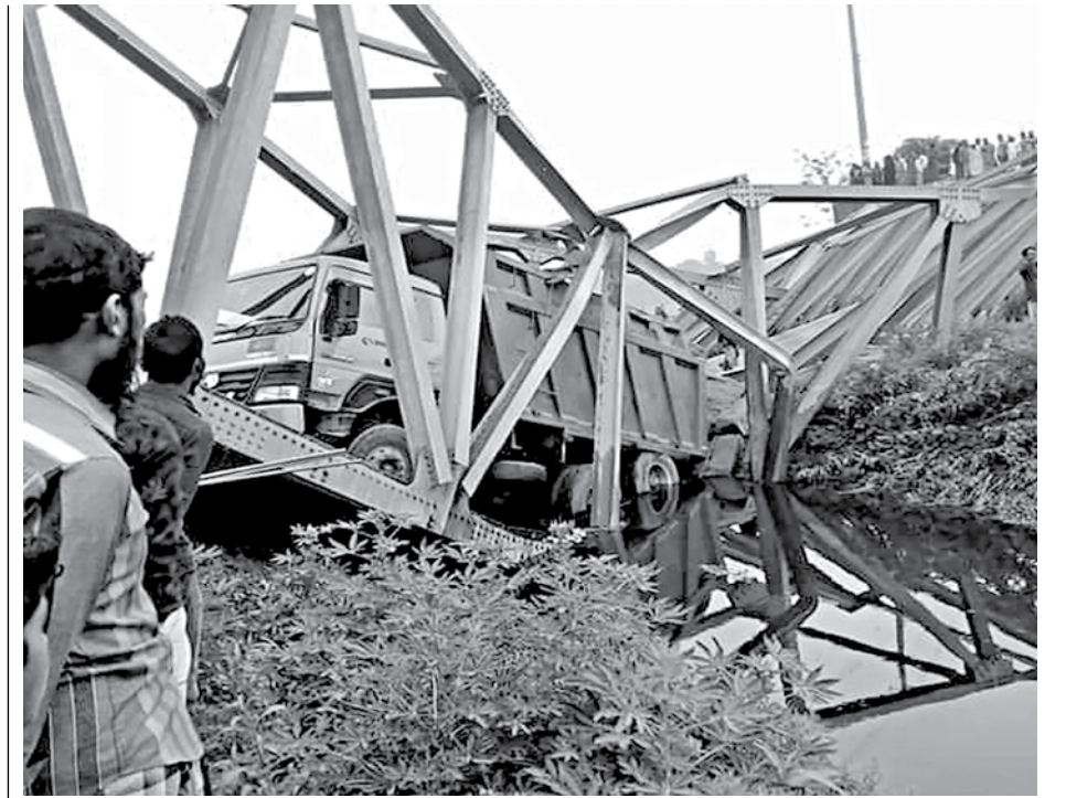
The damaged Bailey bridge on Bhaluka-Mollikbari road in Mymensingh's Bhaluka upazila. PHOTO: COLLECTED
