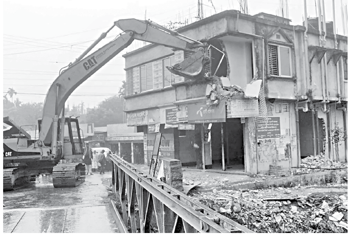
An illegal structure along the bank of the Louhajang river, in Beradoma area of Tangail town, is being dismantled on the second day of drives against illegal occupation of the river's land.
