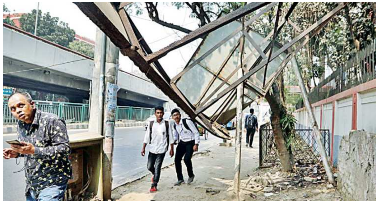
Pedestrians duck as they walk under a passenger shed that has collapsed near the city's Sat Rasta Intersection yesterday. The roof of the shed, which has been in a state of disrepair for some time, caved on Saturday night.
