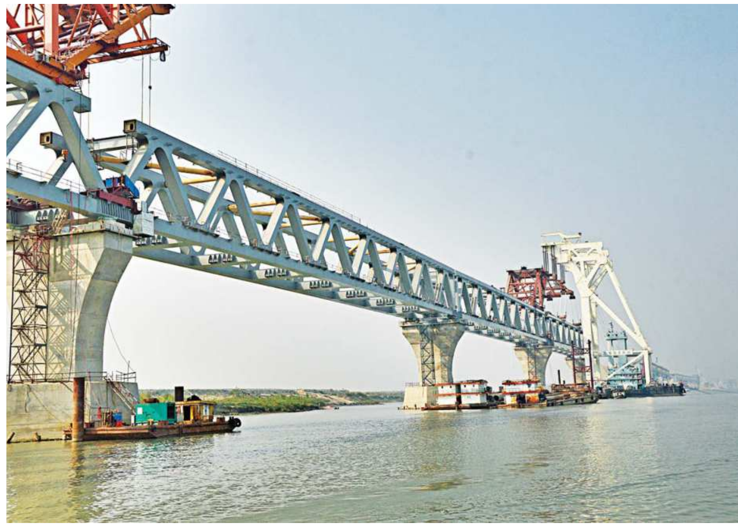
The 25th span of the under-construction Padma Bridge is being installed between its 29th and 30th pillars on the Jazira end of the bridge yesterday. With this, 3.75-km of the 6.15-km bridge has become visible.
