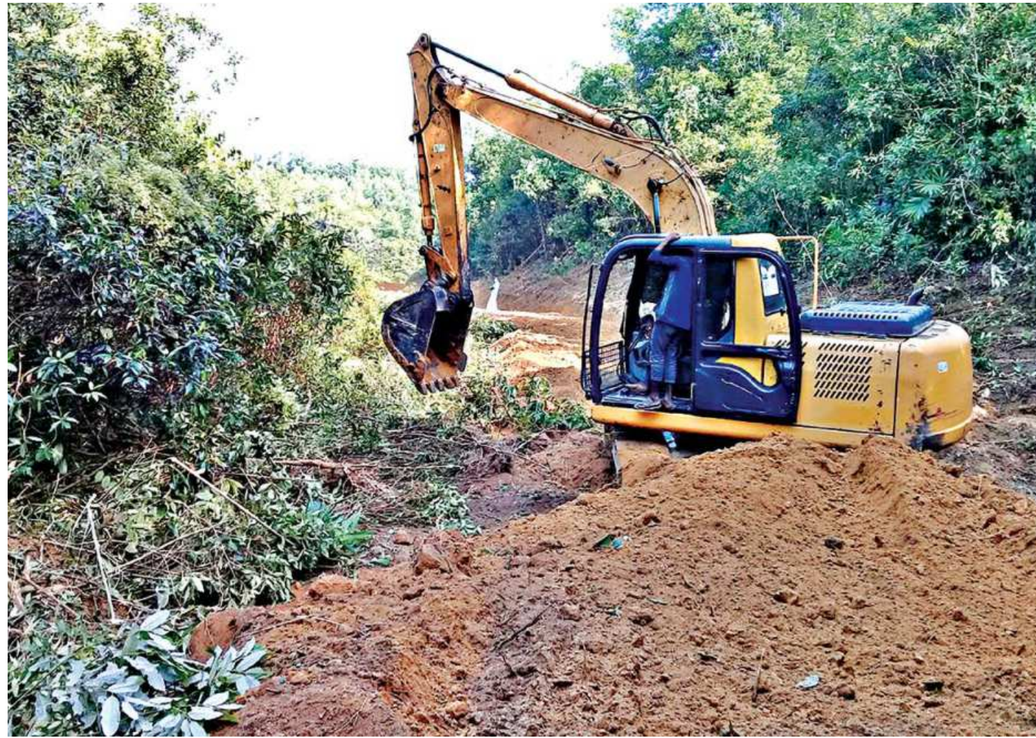
Defying a court order, an excavator, deployed by Halda Valley, clears trees at a hillock at Ramgor-Sitakunda forest in Chattogram's Fatikchhari upazila to make a road. The photo was taken last month.
