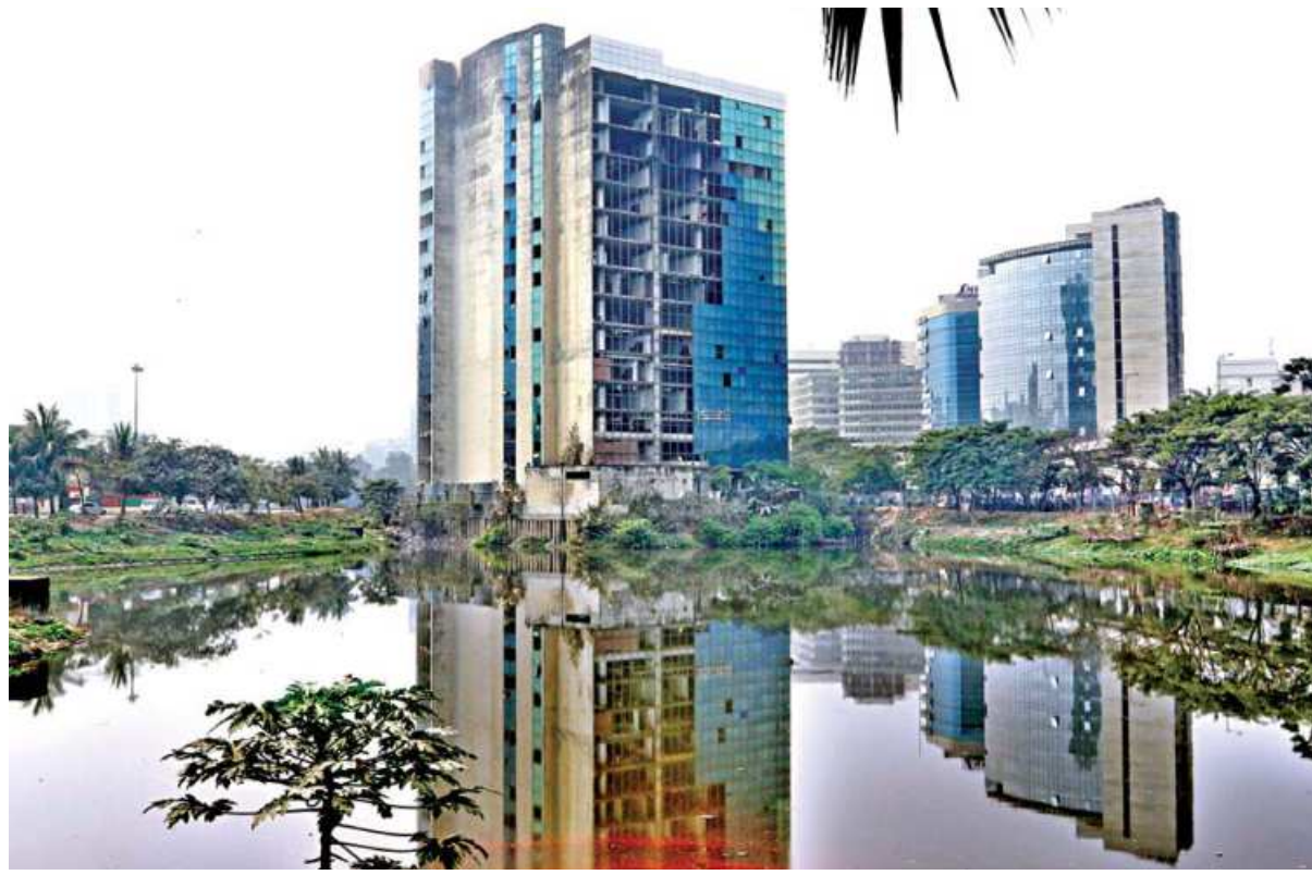
Constructed illegally, the BGMEA building in Hatirjheel still stands, as the demolition work continued at a snail's pace due to lack of power supply. Utility connection was finally restored yesterday and it will be dismantled within six months, said authorities concerned.
