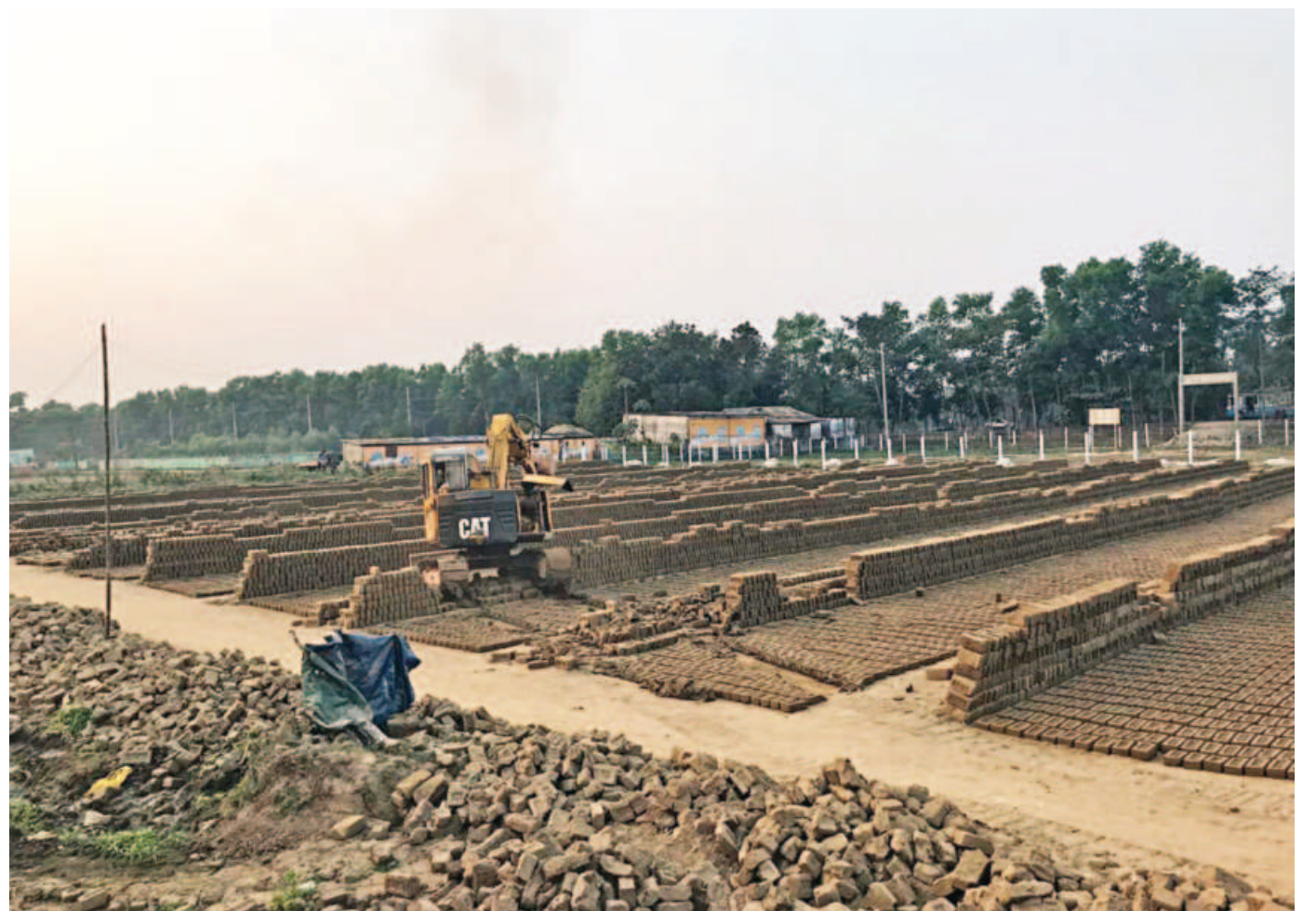
A DoE excavator destroys unbaked bricks at Khan Bricks in Kulaura upazila on Tuesday.
