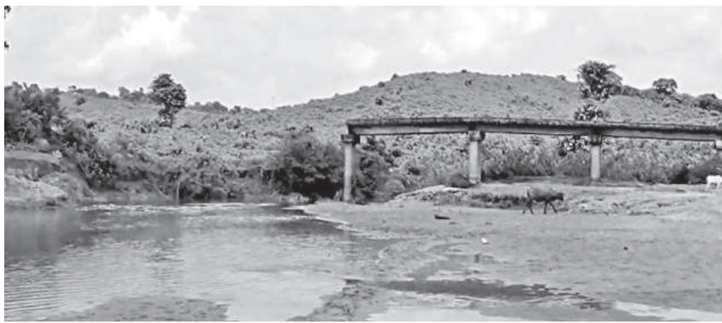
A bridge on a canal in Netrakona's Durgapur upazila lies broken for three years, causing immense sufferings to people.
