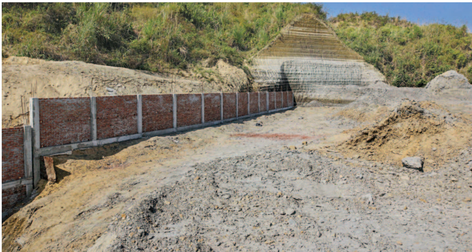
A wall constructed after flattening part of a hill in Jangal Salimpur area of Chattogram's Sitakunda upazila. A construction firm named Spectra Engineering Limited, which razed the hill, claimed it did this to keep construction materials there. The photo was taken on Thursday.
