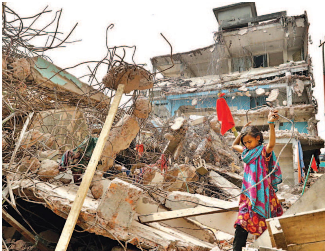
A girl walks on the rubble of a five-storey building, illegally built on the Turag river, after a part of the structure was knocked down by Bangladesh Inland Water Transport Authority during an eviction drive in Tongi's Abdullahpur area yesterday.
