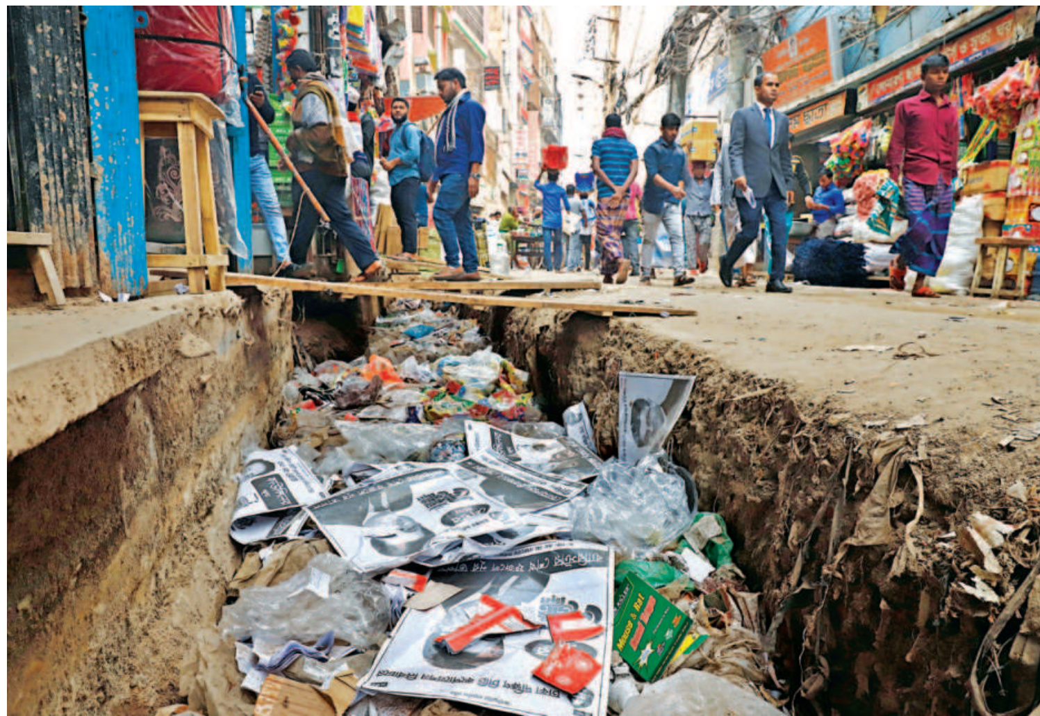
A trench was dug up on this road in Old Dhaka's Chawk Mogaltuli area about two months ago to construct a sewer. The slow progress of the work is causing sufferings to locals as almost half of the road remains unusable. Traders also spend extra money to transport their goods to and from their shops. The photo was taken yesterday.
