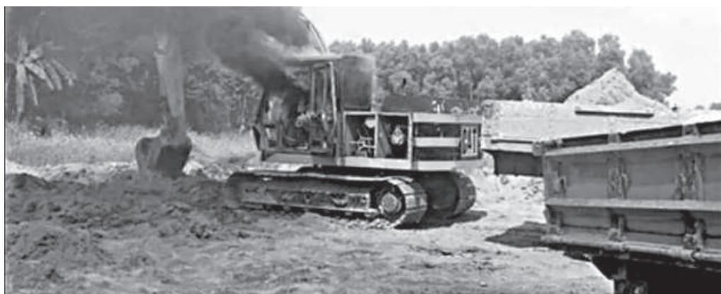
An excavator that was used to lift sand from the Jhinai river in Tangail's Basail upazila was burnt yesterday during a mobile court drive.
