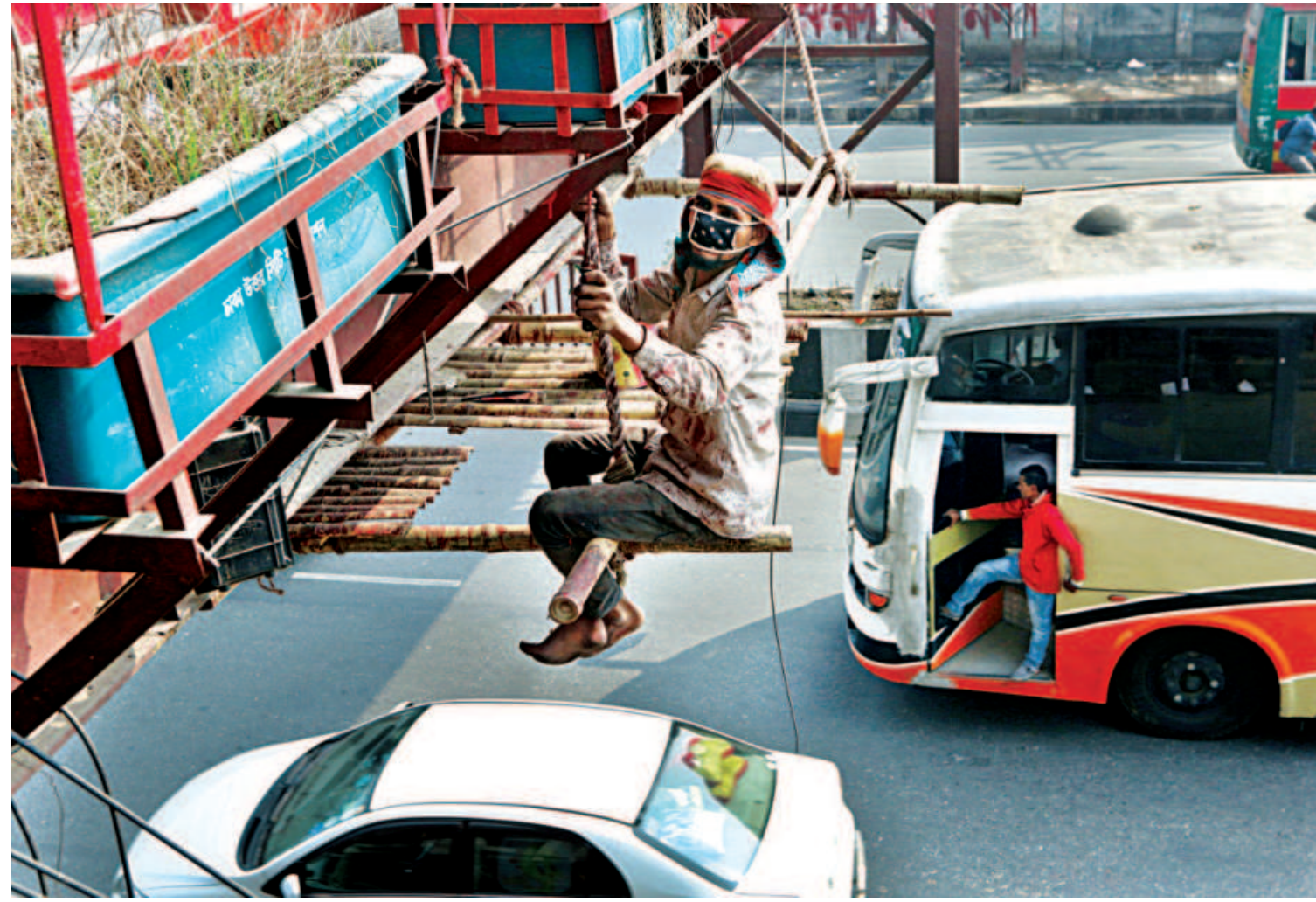
With no safety gears, a worker dangles from a makeshift rope ladder while painting a footbridge in Darussalam area of the capital's Mirpur. He runs the risk of falling to the busy street below and getting hit by vehicles. The photo was taken a couple of days ago.
