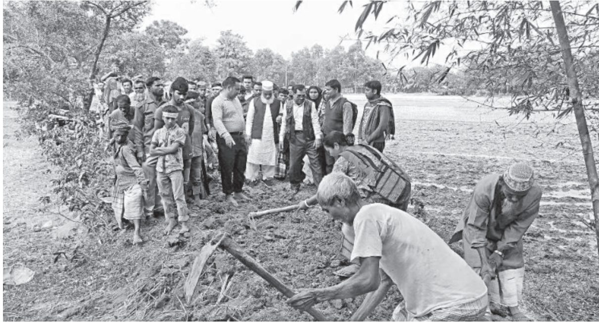
People of all ages join hands to repair this three kilometre road in Lengura union in Netrakona's Kalmakanda upazila yesterday. They took the initiative after repeated appeals to the authorities concerned fell on deaf ears.
