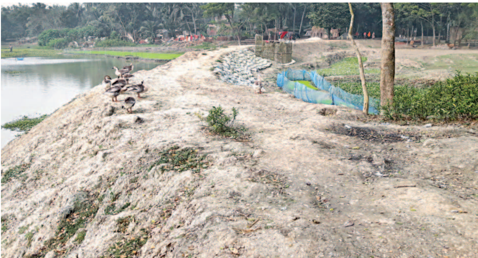
Embankment built at the mouth of Sonalidanga canal in Jhenidah's Kaliganj upazila impedes flowing down of water from the adjacent Majdia beel, eventually inundating a large area of croplands in the area.
