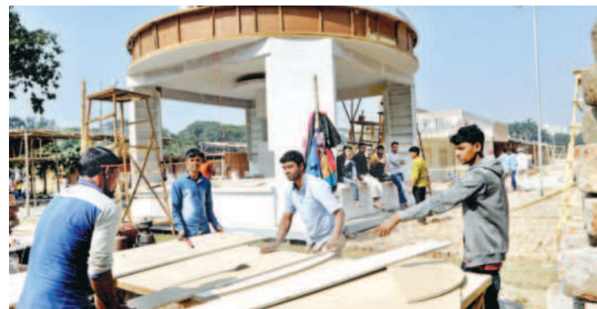
Workers set up a pavilion for Amar Ekushey book fair in Suhrawardy Udyan yesterday.
