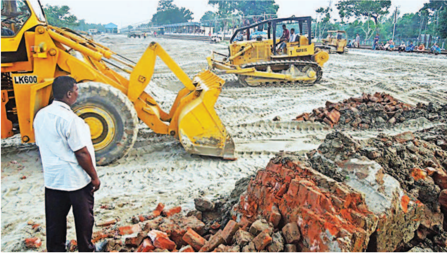
Work is going on in full swing to construct the rail track from Nilphamari's Chilahati station to the Indian border as the authorities concerned are expecting inauguration of the third direct train communication with the neighbouring country by July this year. PHOTO: EAMASADUZZAMAN
