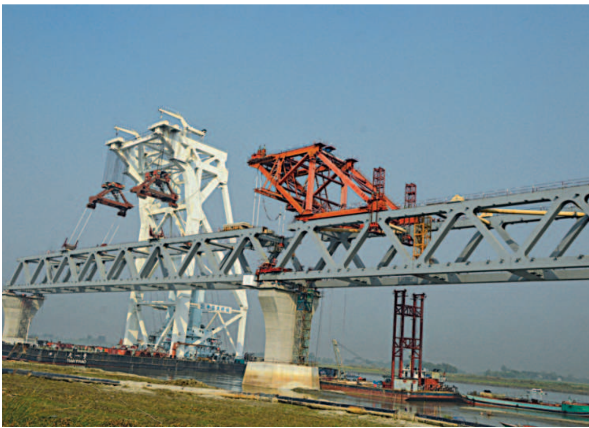
The 21st span of the under-construction Padma Bridge is placed between the 32nd and 33rd pillars of the bridge at Jajira point of Shariatpur yesterday. With this, 3.15 km of the 6.15 km bridge has now become visible. PHOTO: STAR
