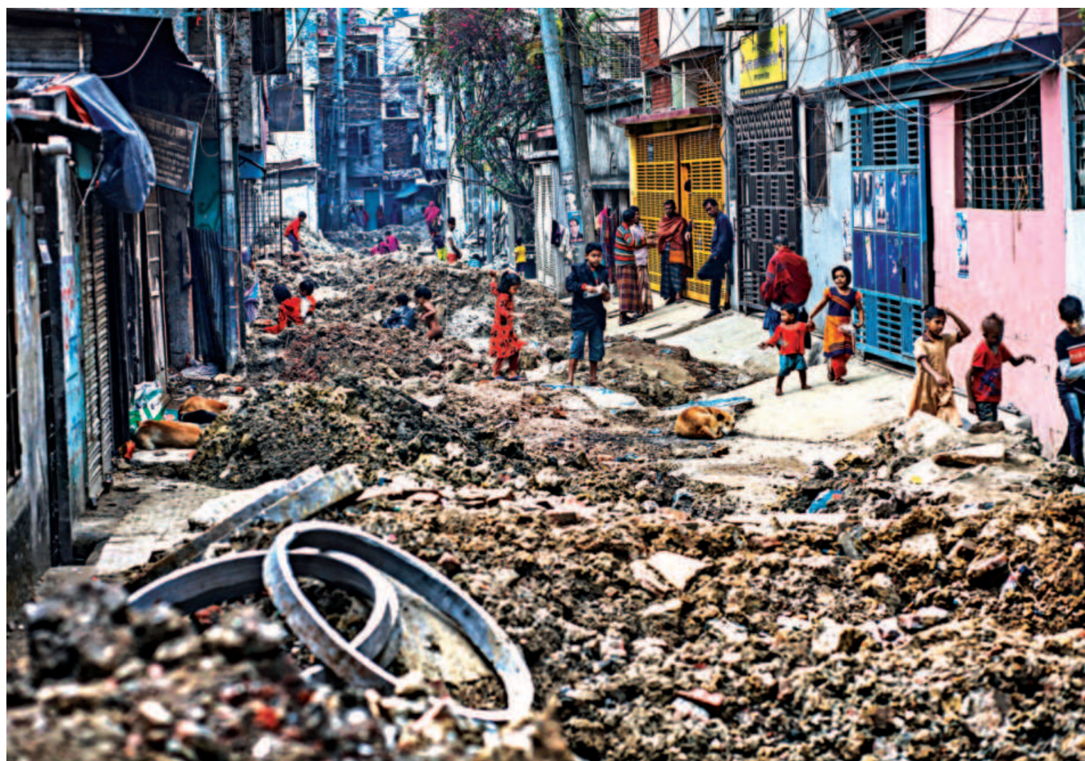
The Madrasa Road-2 in the capital's Muhammadpur has been rendered useless as Dhaka North City Corporation works on the sewer lines. Residents of the area said they had been subjected to the suffering for eight days with no transport able to reach their homes. Their vehicles are either stuck in the garage or have been parked elsewhere.
