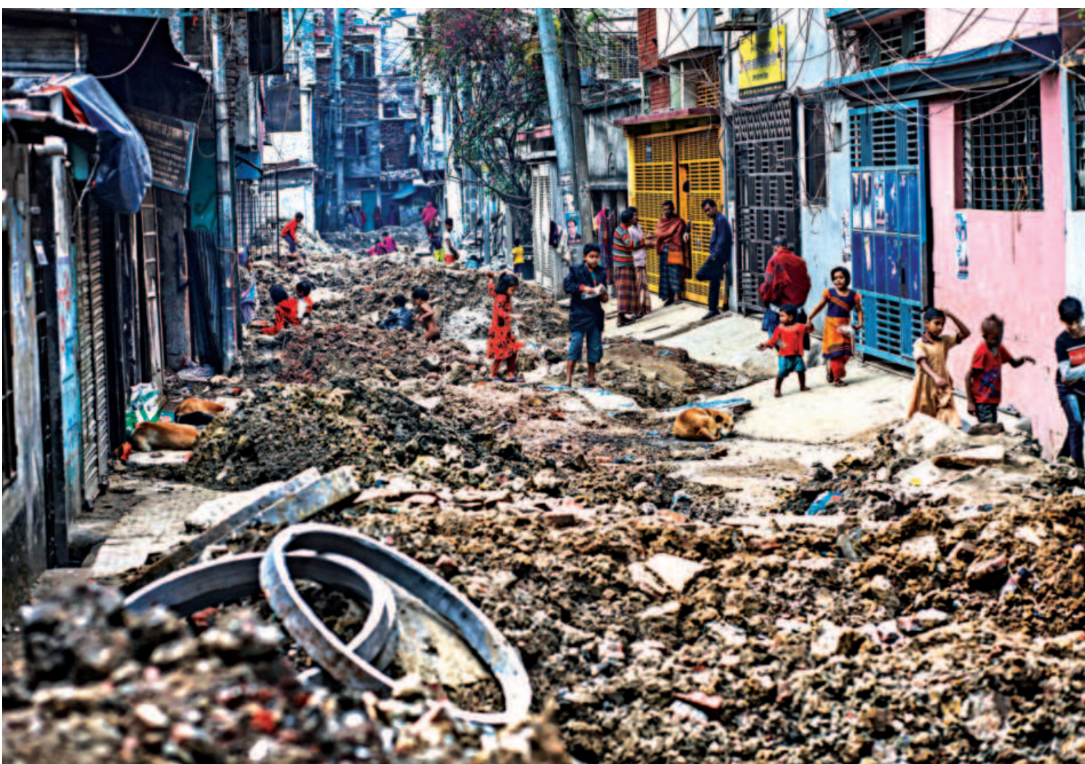
The Madrasa Road-2 in the capital's Muhammadpur has been rendered useless as Dhaka North City Corporation works on the sewer lines. Residents of the area said they had been subjected to the suffering for eight days with no transport able to reach their homes. Their vehicles are either stuck in the garage or have been parked elsewhere.
