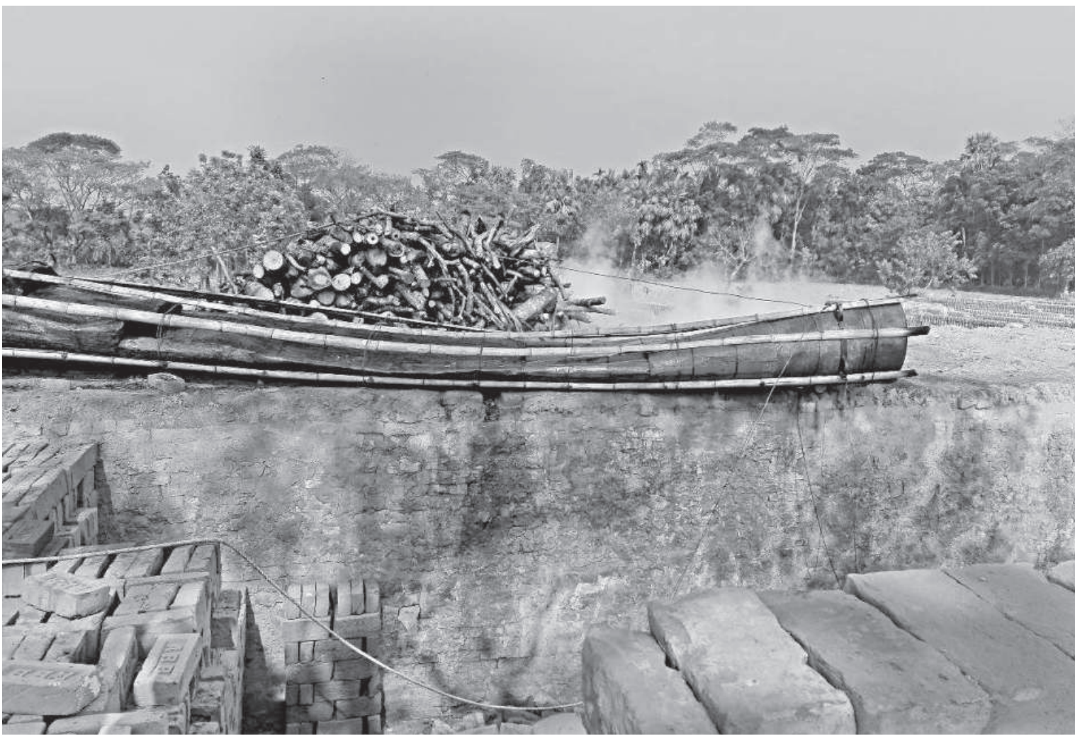
DoE in a drive dismantled four illegal brick kilns in Barishal on Thursday.
