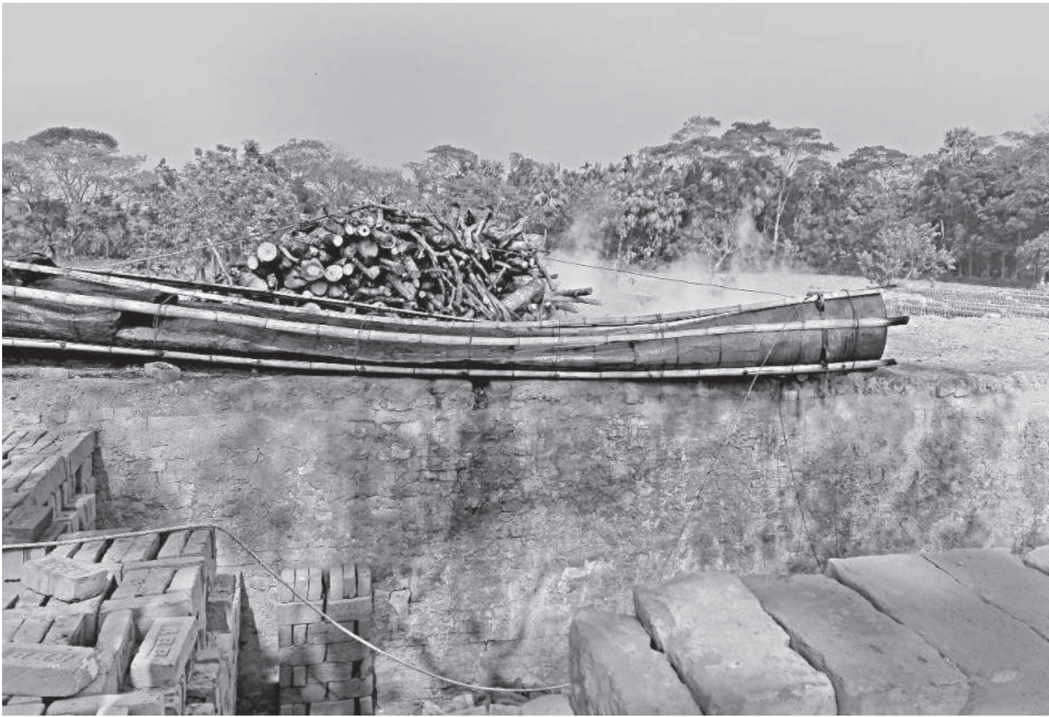
DoE in a drive dismantled four illegal brick kilns in Barishal on Thursday.
