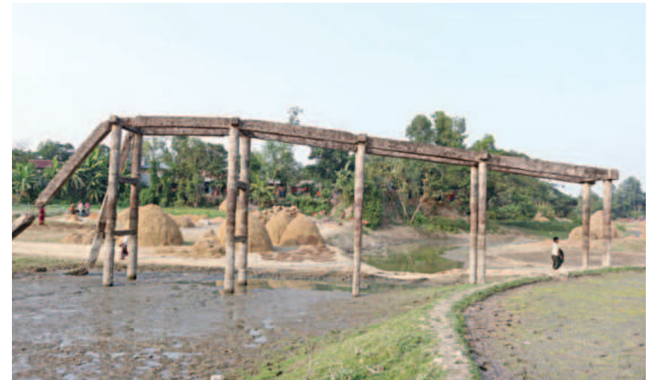
The bridge was destroyed by floods of 1988 and since then no new bridge has been built there, leaving thousands of commuters in great trouble of Brahmanbaria's Nasirmagar upazila.
