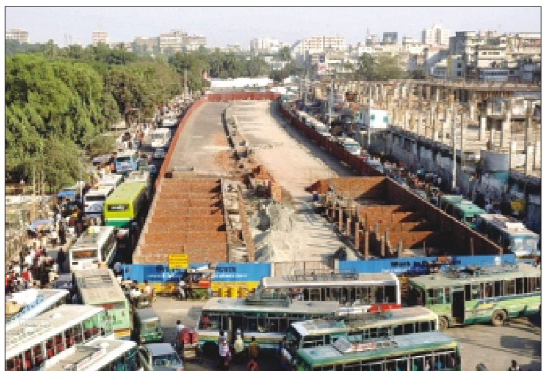
Site offices for the Gulistan-Jatrabari flyover at Gulistan in the capital are being built on the middle of the road narrowing the already congested intersection.
