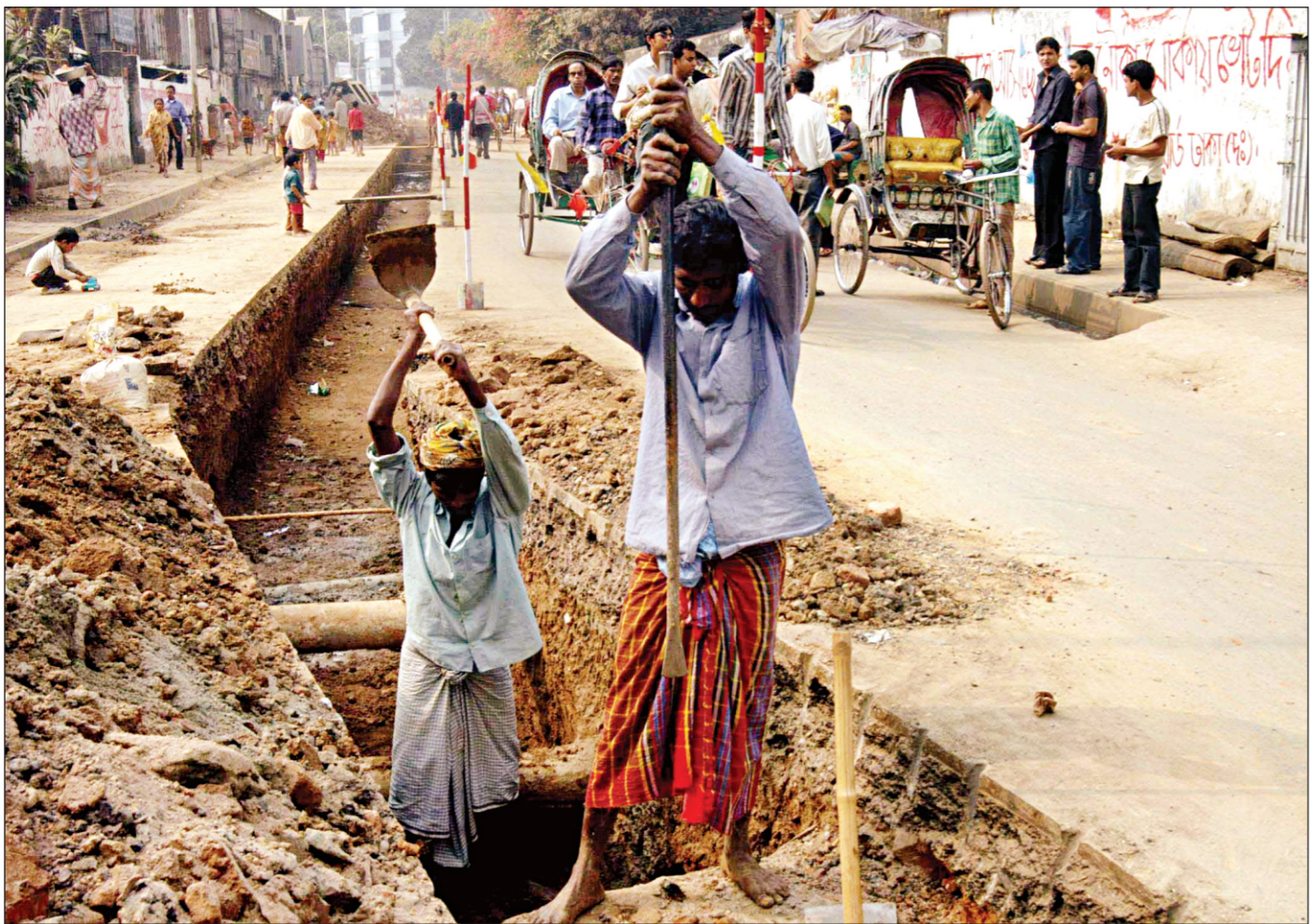
Along trench is being dug in the middle of a road at Paribagh in the capital to install power cables, ignoring pedestrians' safety as the road is still open to public.
