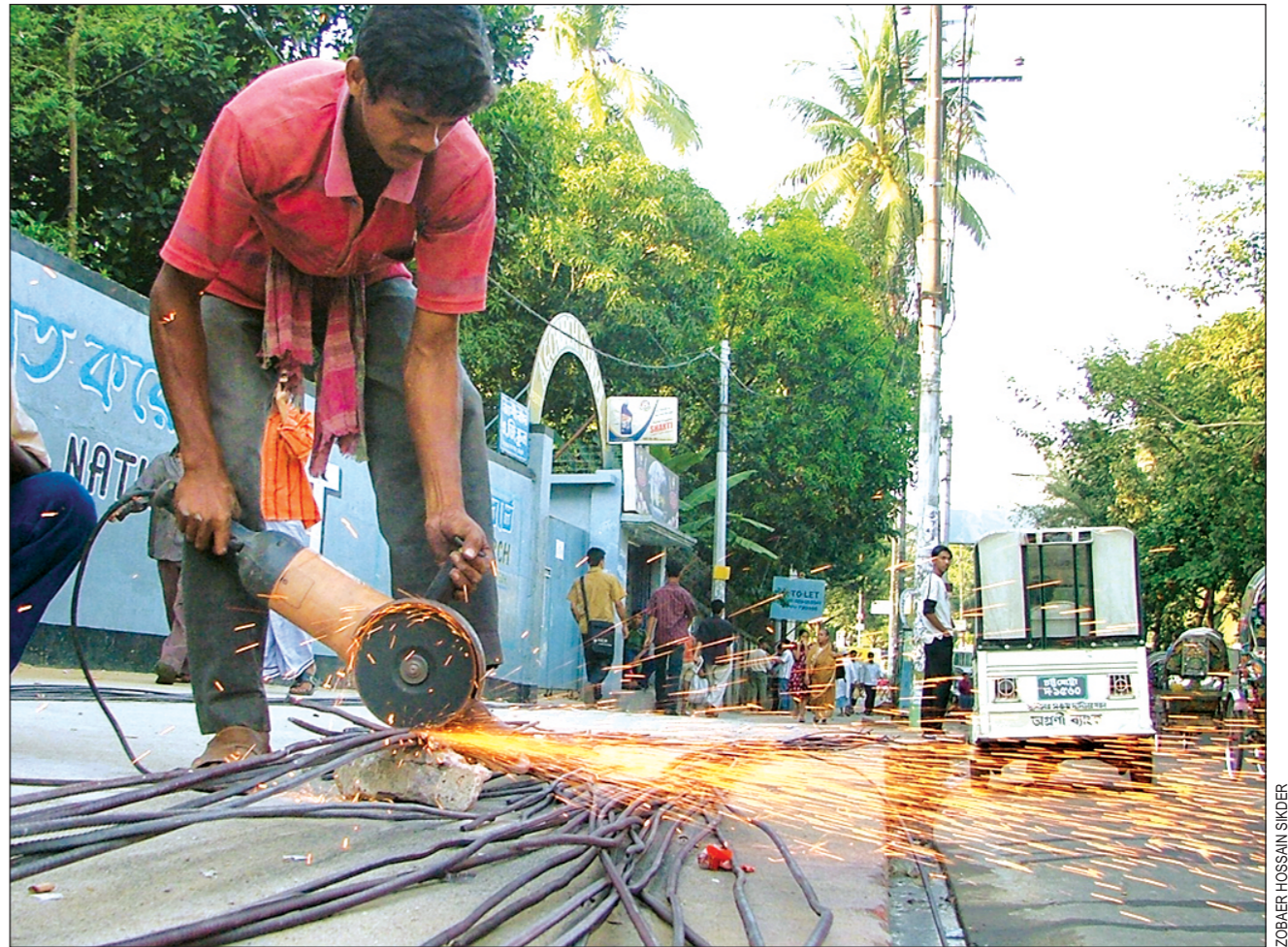
A construction worker cuts iron rods on a sidewalk in front of a kindergarten school at Jamal Khan, posing danger to schoolchildren as well as passers-by, but the authorities turn a blind eye to the menace.
