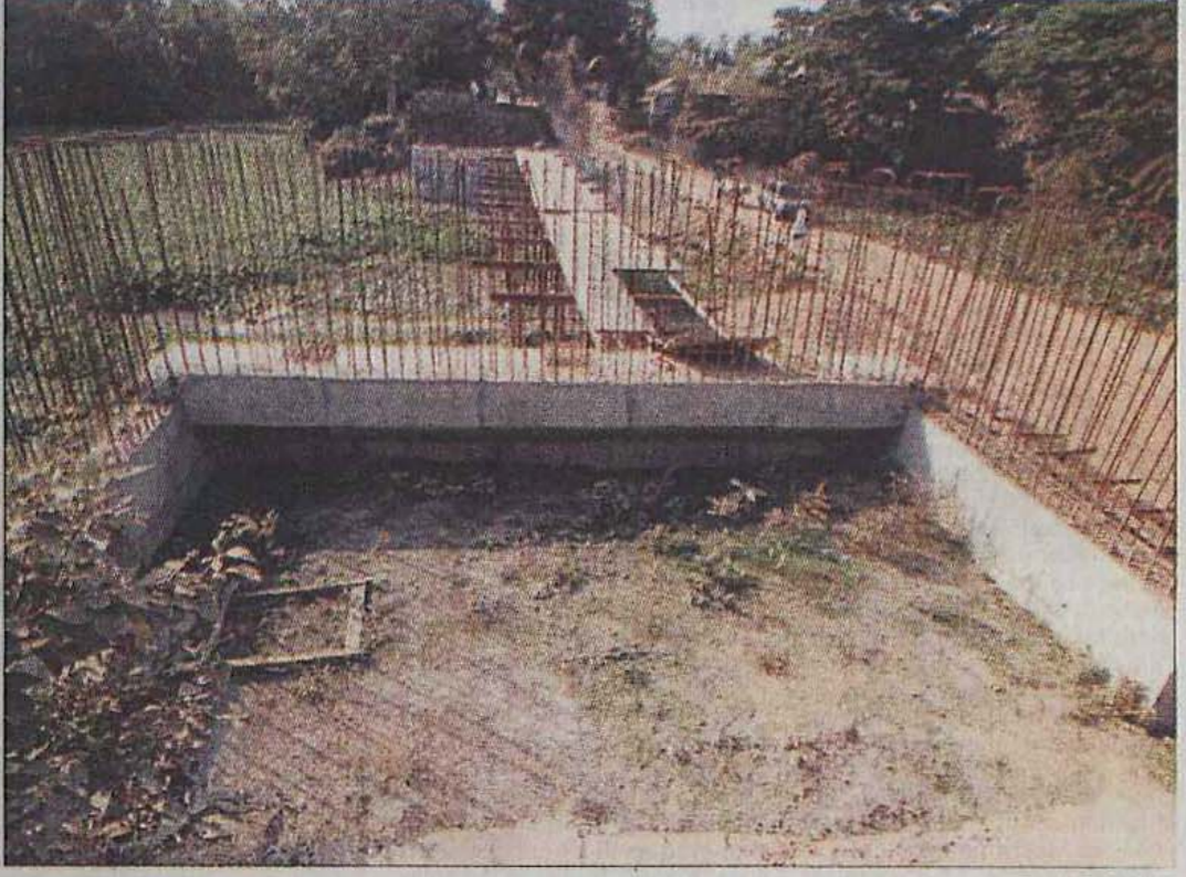
The bridge at Dholla on Hemayetpur-Singair road on the outskirts of the capital lies incomplete, obstructing traffic movement. Its construction started almost a year ago under an emergency rehabilitation project after flood damage.
