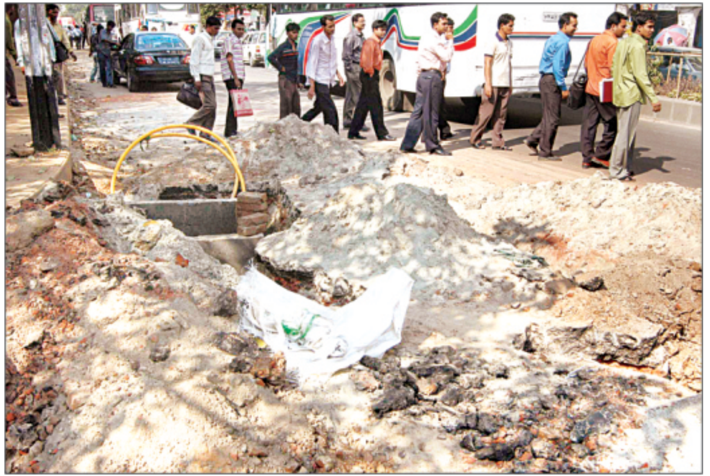
Authorities have turned a blind eye to the suffering of commuters and pedestrians caused by road digging from Science Laboratory to High Court intersection in the city. The road was dug for installation of underground cables, but no steps have been taken to repair the road on urgent basis.
