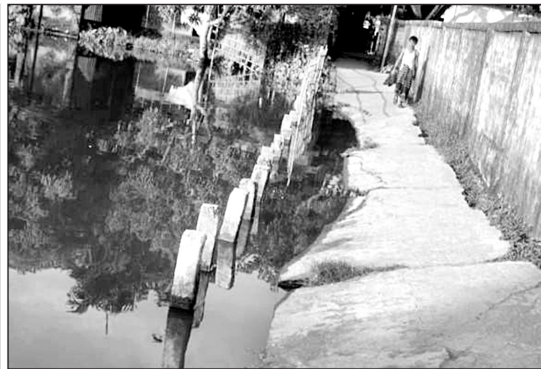
Flood damaged Post Office Road in Derai upazila of Sunamganj. The road is yet to be repaired although 3 years passed after the deluge. PHOTO: STAR
