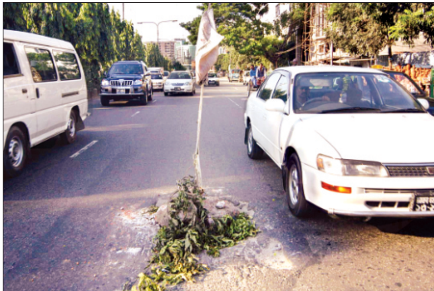
A bamboo pole is all there to warn passing vehicles and pedestrians as a manhole with no cover on Mirpur Road in the city poses danger.
