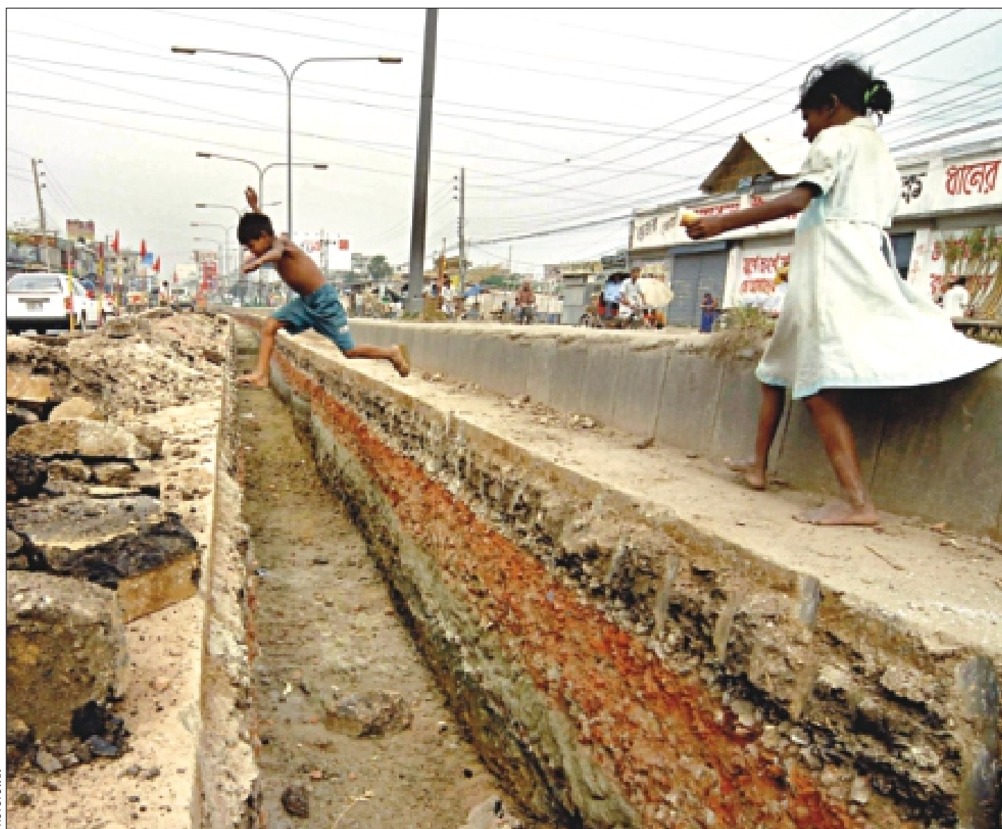
Power Grid Company of Bangladesh installing underground cables digs a long trench on the fast lane of the street near Rampura bridge in the capital and puts the rubble on the road, creating hazards to passing vehicles.
