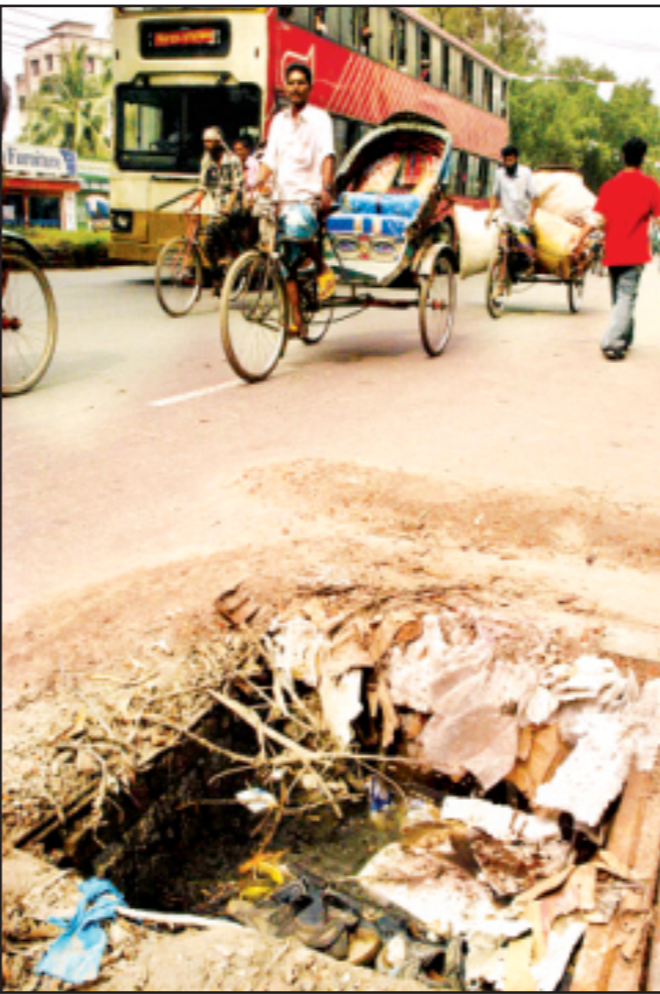
PHOTO: STAR A run-down manhole with no cover in the middle of a road at Rokeya Sarani, Shewrapara, in the city poses danger to pedestrians as well as passengers.
